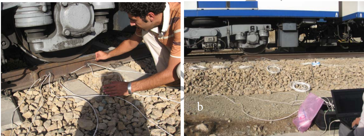
Figure 5 (a) the location of strain gauges (b) moving train on installation location of strain gauges during the tests
